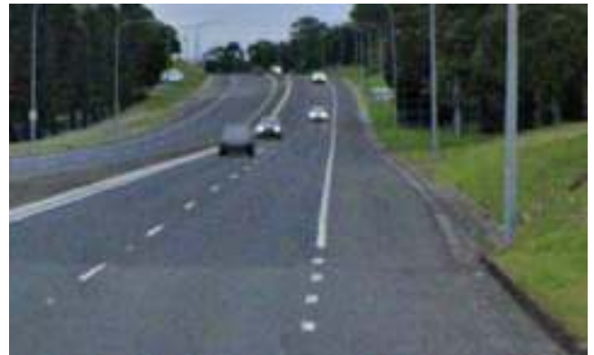
▲ Inadequate markings on the shared path and drop of cycle shoulder
