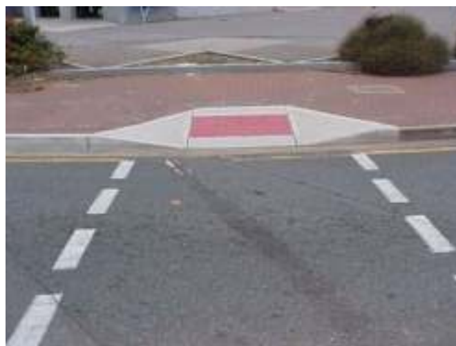
▲ Example of a compliant kerb ramp
