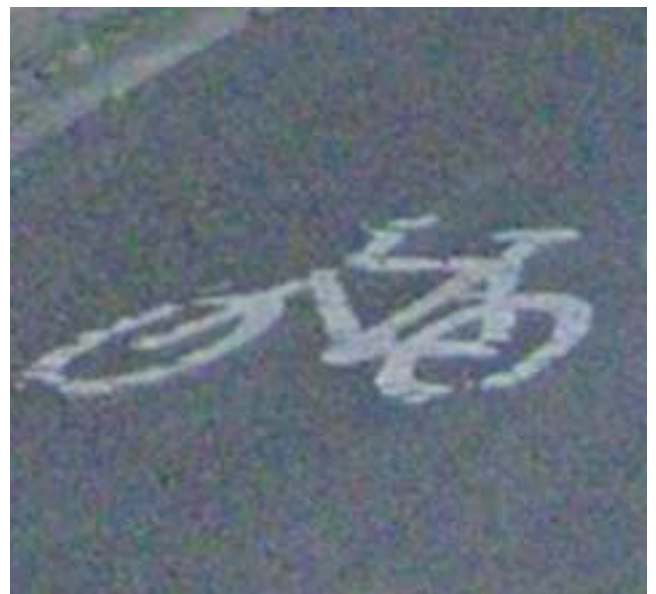
▲ Old road markings on shoulder are fading
