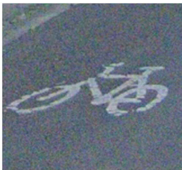
▲ Old road markings on shoulder are fading
