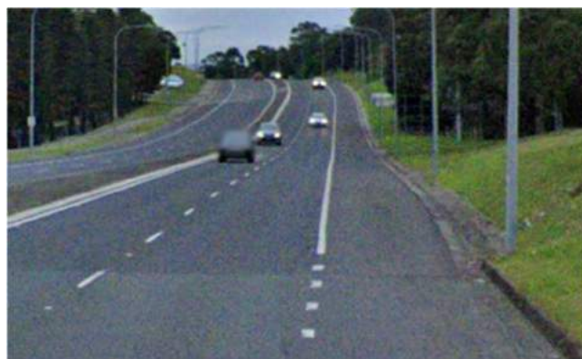
▲ Inadequate markings on the shared use path and drop of cycle shoulder
