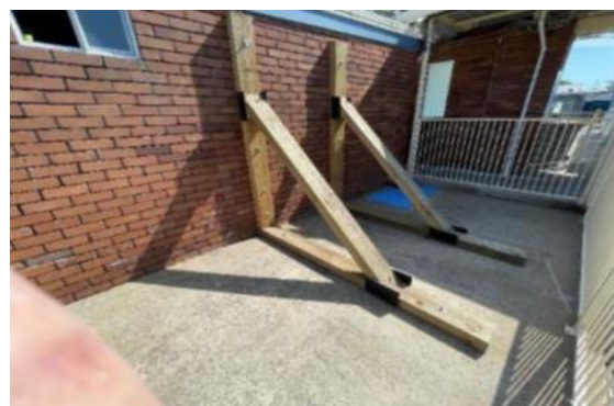
Oak Flats 25m pool Plant Room
