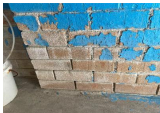
Albion Park Pool Chemical Bunding
